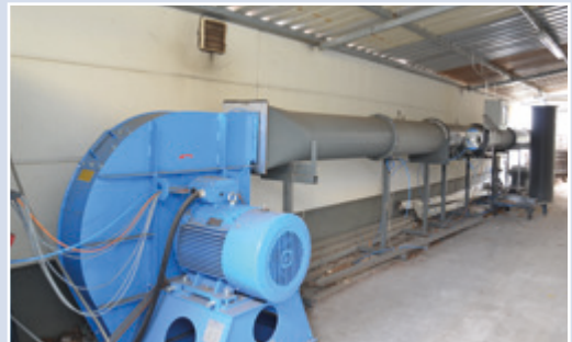
Test station at JASTA-ARMATUREN
